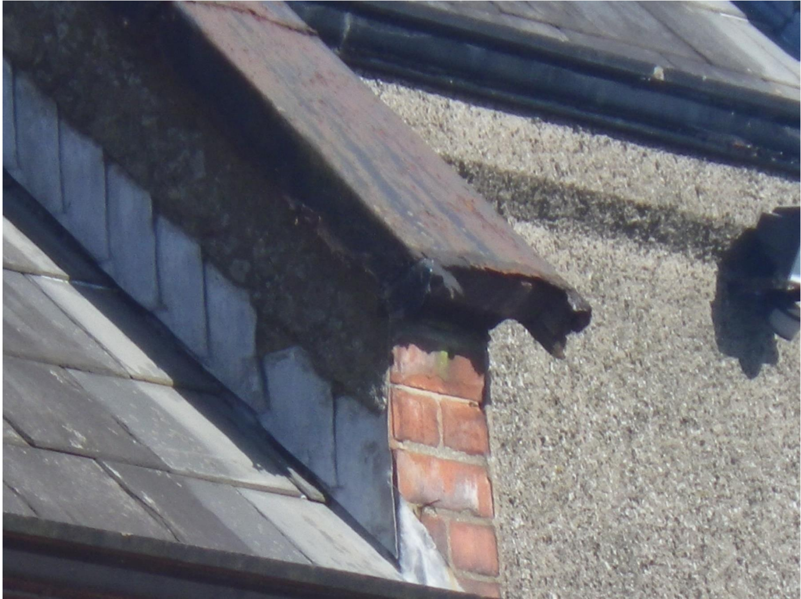
Failing metal covers to verges
