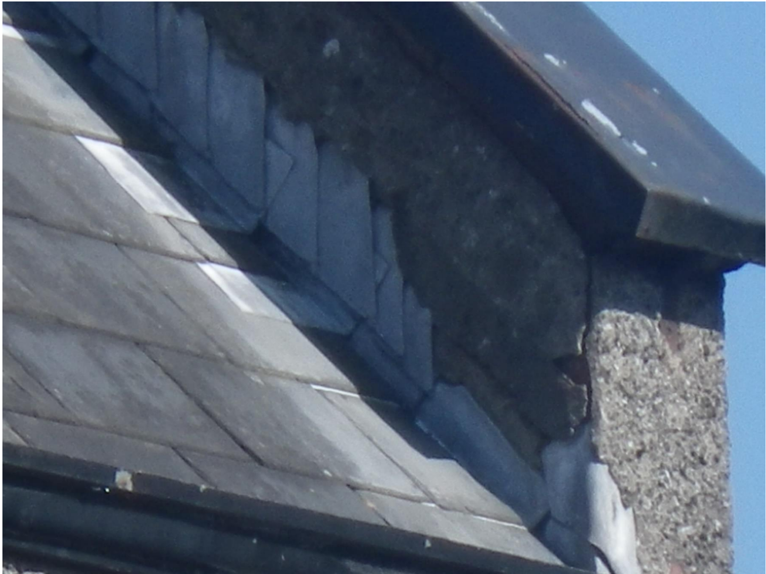
Failing lead detail at Chancel roof abutment
