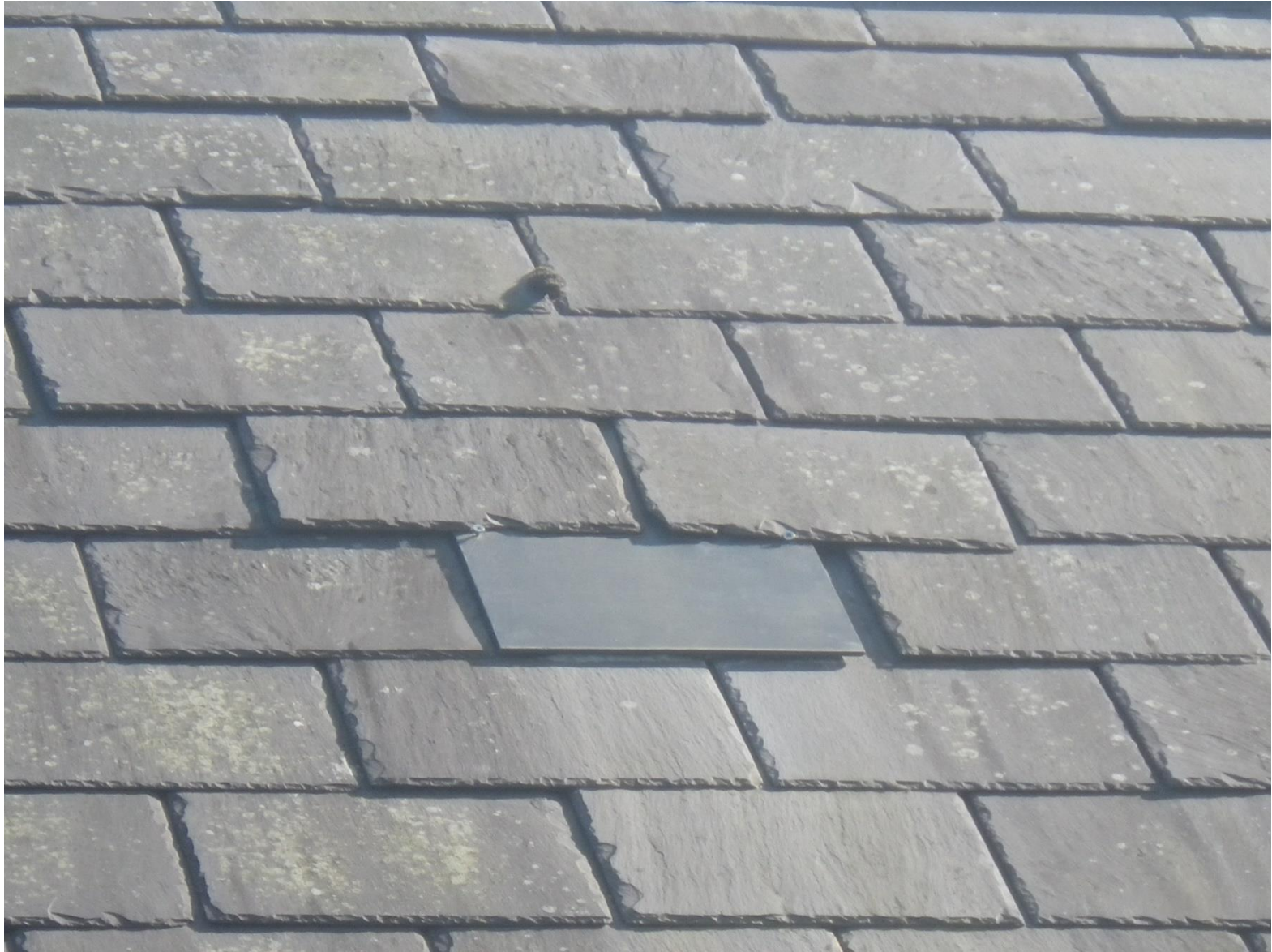
Poor replacement slate
