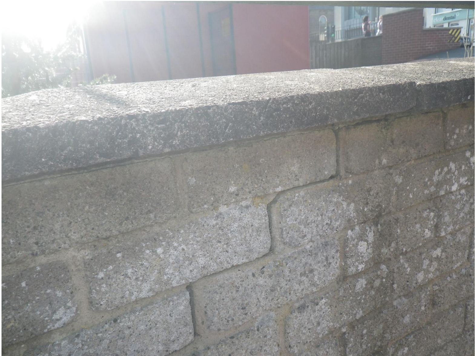
Loose brickwork to boundary wall
