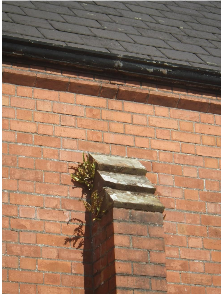
Vegetation growing to south wall pier
