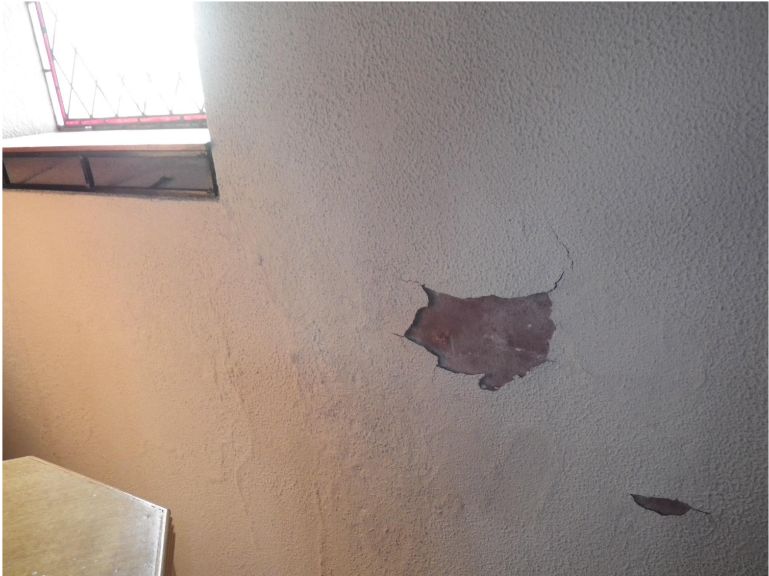
Residual dampness to Nave wall
