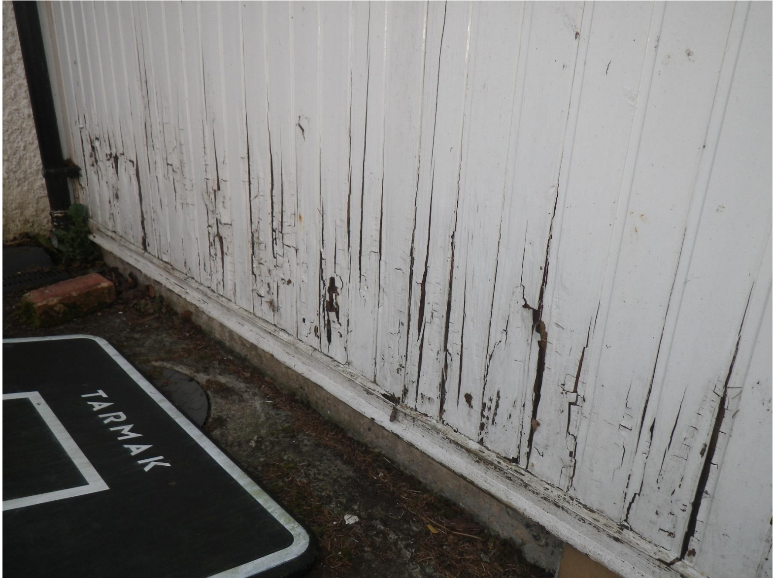
Timber decay to cladding at Utility Room
