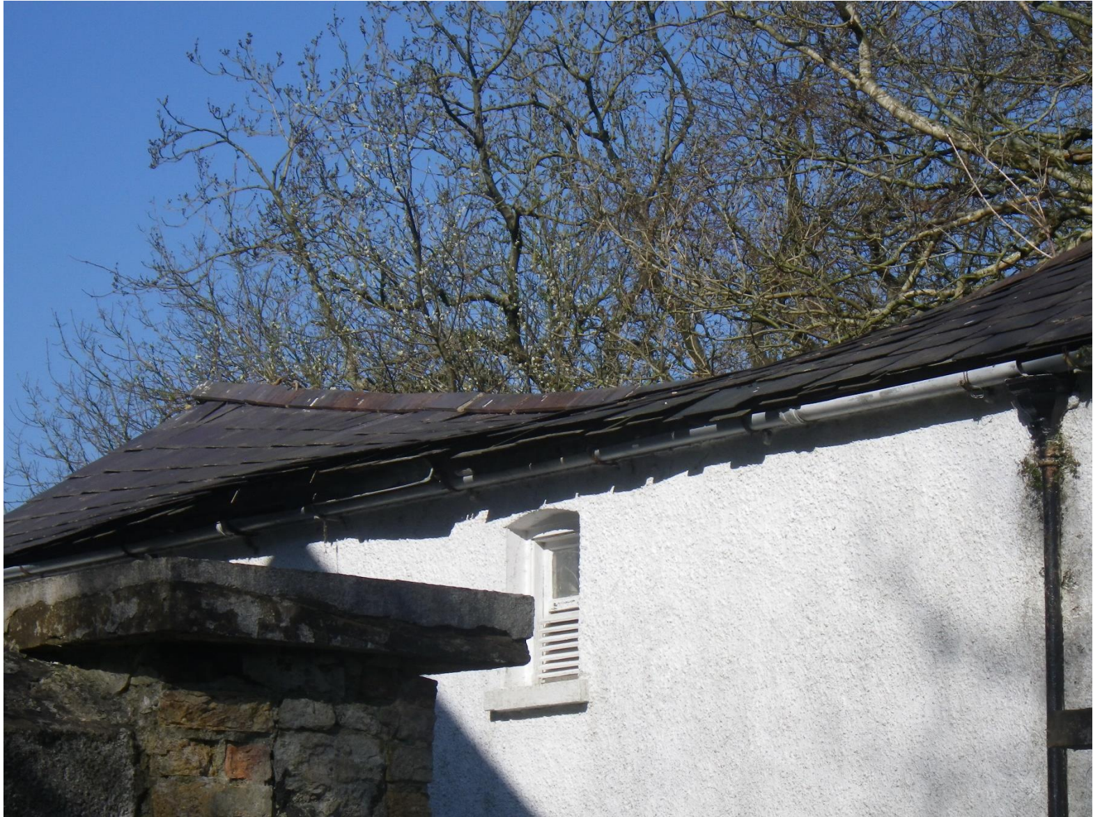
Dangerous condition of Outbuilding.
