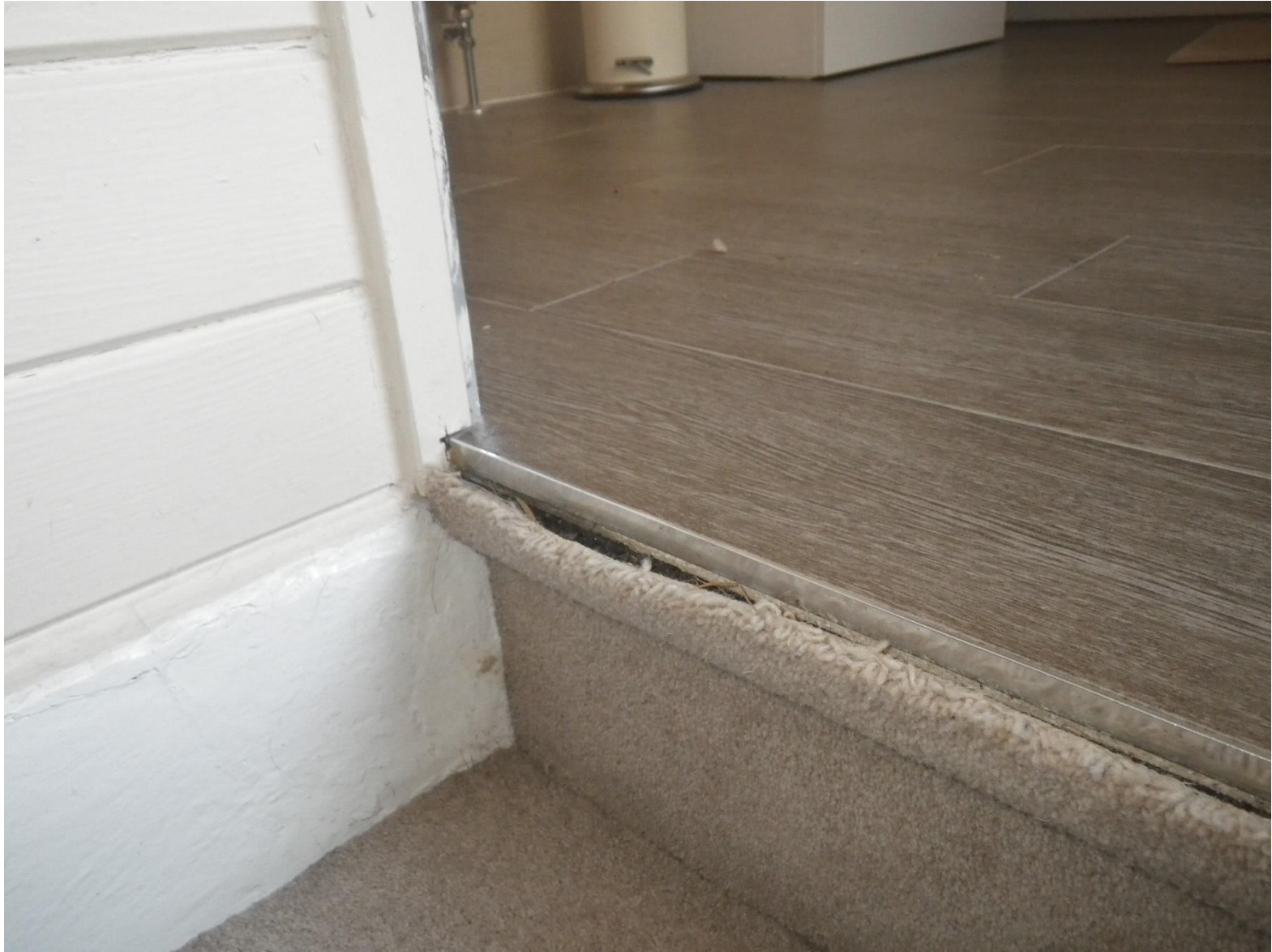
Trip hazard to Bathroom door threshold
