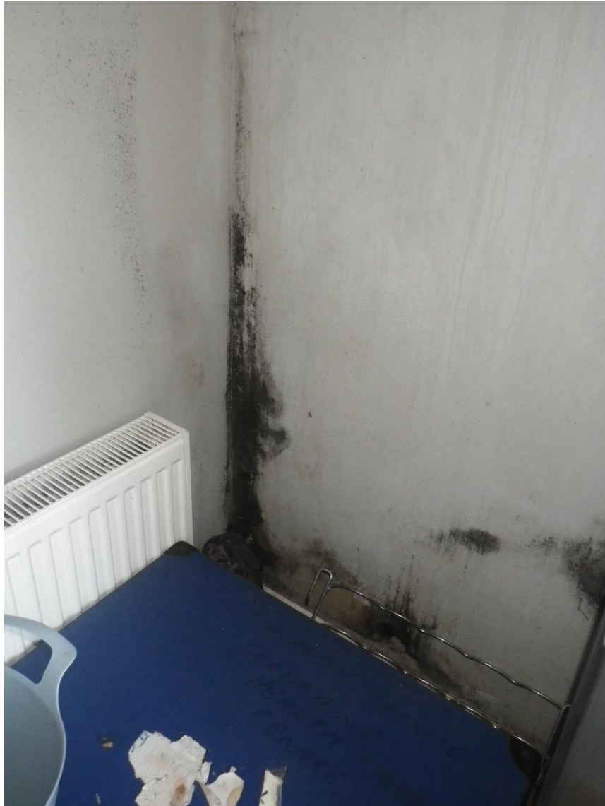
Heavy condensation to Utility Room
