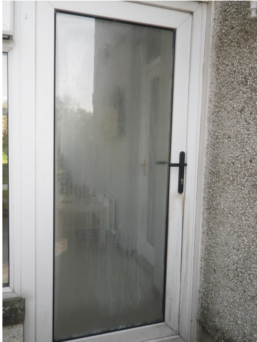
Example of extensive condensation to double glazed units
