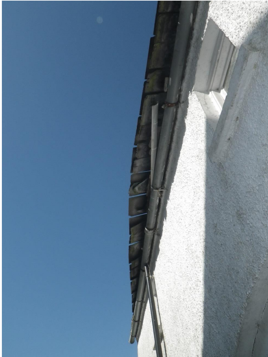
Risk of falling slates outbuilding roof
