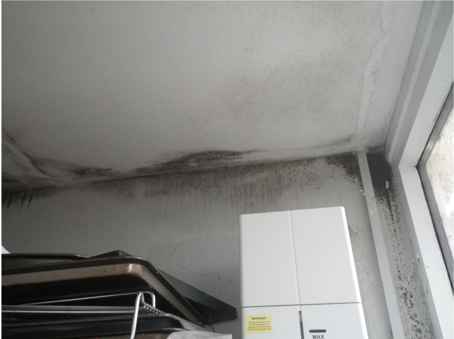
Heavy condensation to Utility Room
