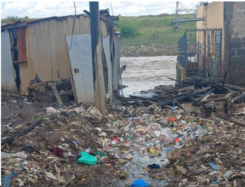
Collapsing house on the banks of a river that had been diverted, where a rubbish dump has arisen and very poor people have settled.
