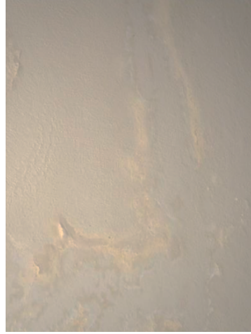
Dampness on West Wall
